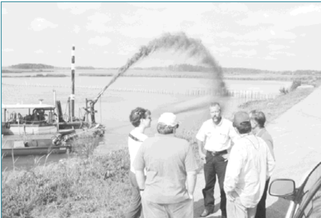
A self-propelled swing-ladder dredge with high-pressure spray nozzle, similar to the one that will be used in the Big Egg Marsh Restoration.
