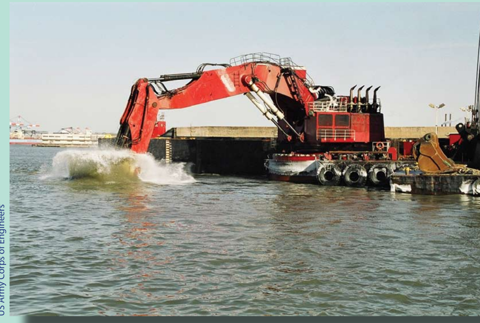
Dredging operations are routine in the Ports of New York and New Jersey.
